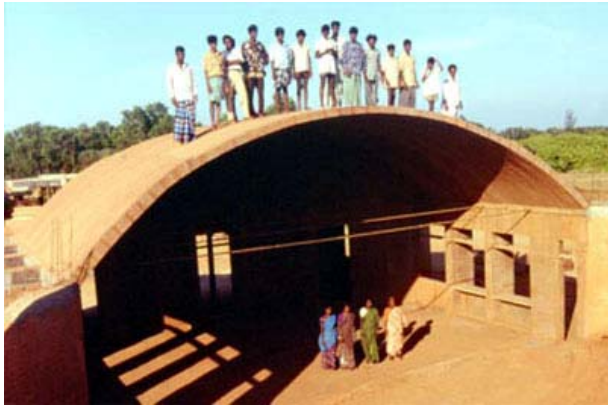
Segmental vault completed in 3 weeks with 4 masons - 10.35 m span, 2.25 m rise. ~ 30 tons, build with the free spanning technique
