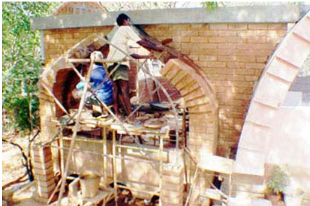
Building a bucket pointed vault, 2.4 m span, with the free spanning technique
