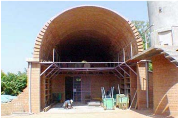
Semicircular vault built free spanning in 37 days with 4 masons - 6 m span, 11 m long, ~ 40 tons
