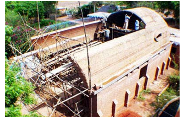
Building a semicircular vault, 6 m span, 11 m long with free spanning technique
