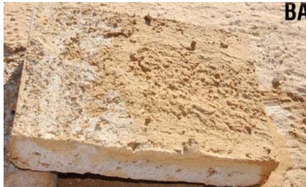
Very good result of water drip test on adobe Ref. BA
