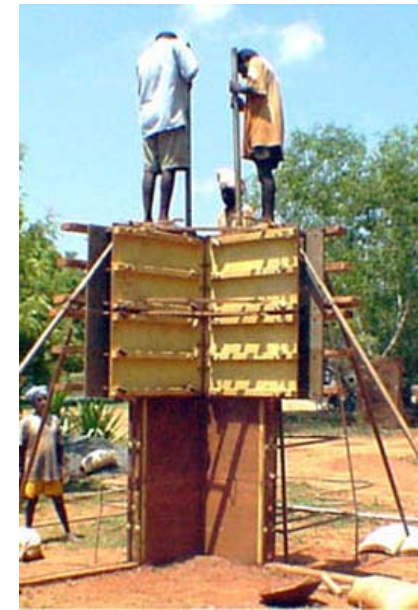
Rammed earth corner form for doing L walls Of L 74/100 cm side & 240 cm high
