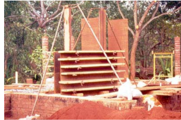
Rammed earth form 224 for doing walls of 99 to 224 cm long & 240 cm high
