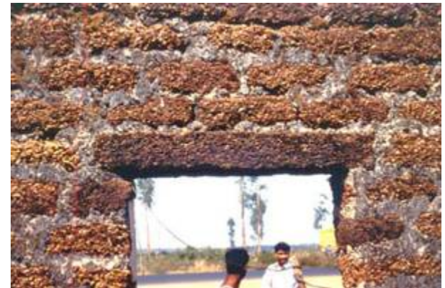
India, Orissa, Near Bhubaneshwar – Lintel ~75 cm span
