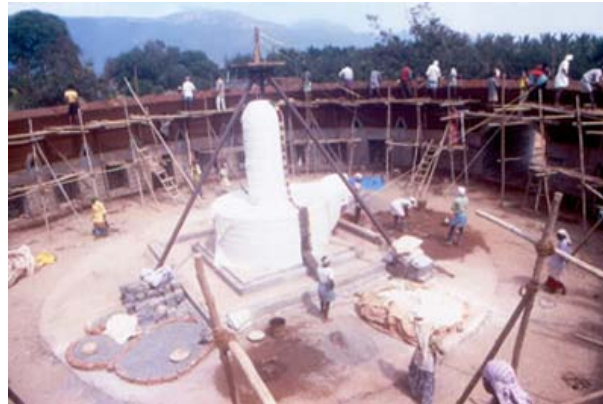
Dome with the Linga and the ropes to check the elliptical shape
