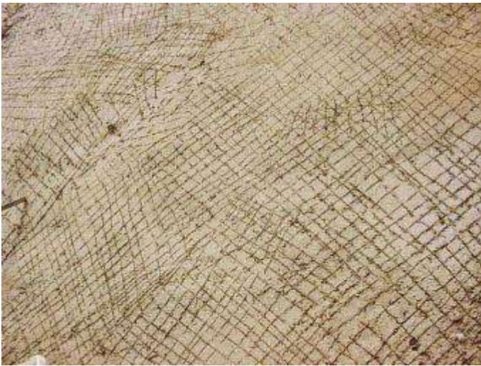
Scratch on the first layer of roof plaster
